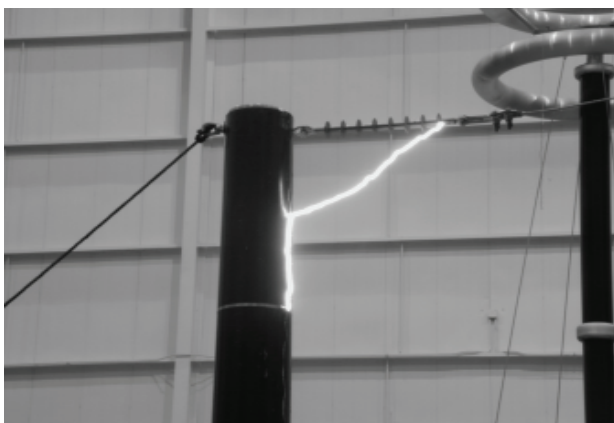
Fig. 3. The 35 kV polymer suspension insulator plus fiberglass pole, the tested pole length is 2 feet. The discharge took place in the air and on the surface of the pole
