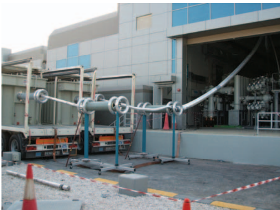
Fig. 4b. Parallel setup of two resonant test systems for testing a 10-km 220-kV cable installation
