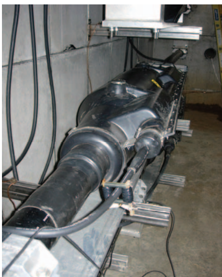
Fig. 3. Photo of HFCT sensor in MH #2
